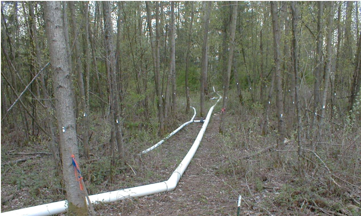
Figure 2 - 27. Manifold and branches in a wooded, vegetated spray field
